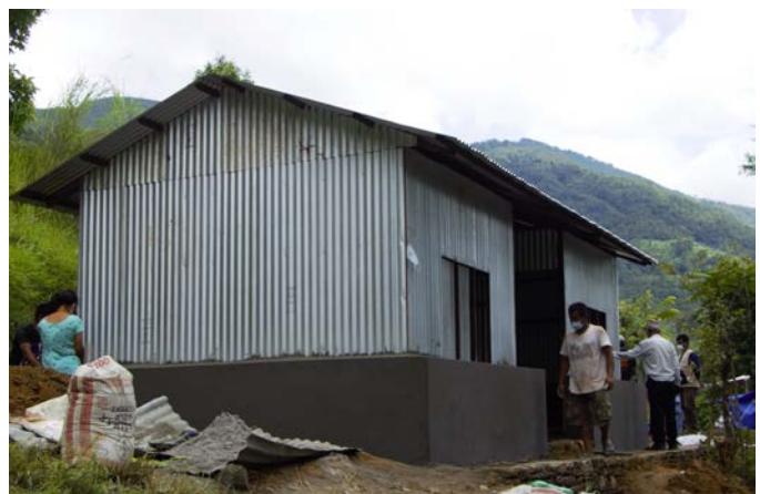
CARE supported flood affected communities in Sindupalchowk to construct transitional shelters which will decrease the risk of COVID-19 as they had been staying in temporary camps.
